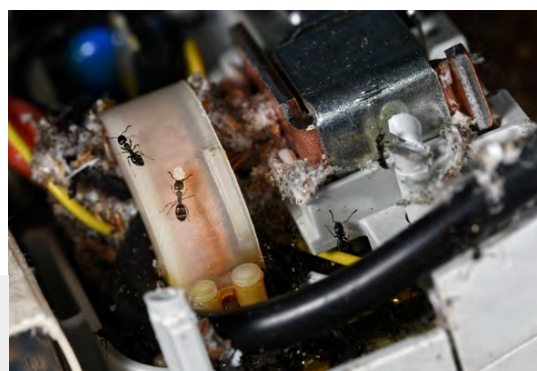
Photo 2. Ochetellus glaber (2.5 mm) nesting in a ruined circuit breaker
