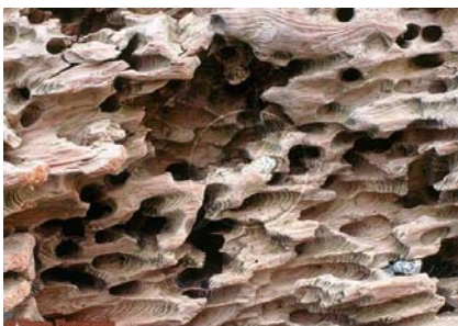
Shipworm-related damage to wood.
