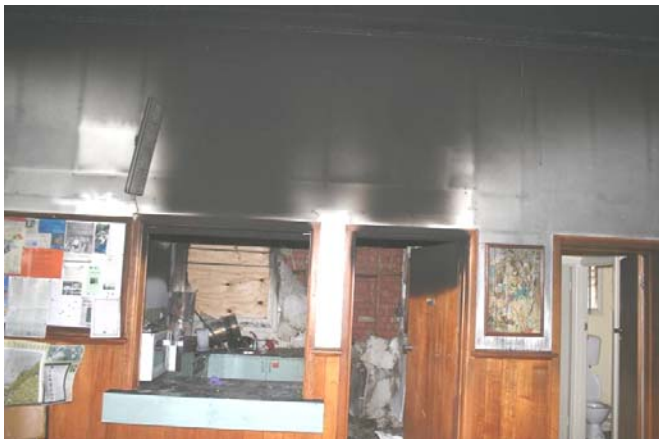
Fire damage— FNCV kitchen
